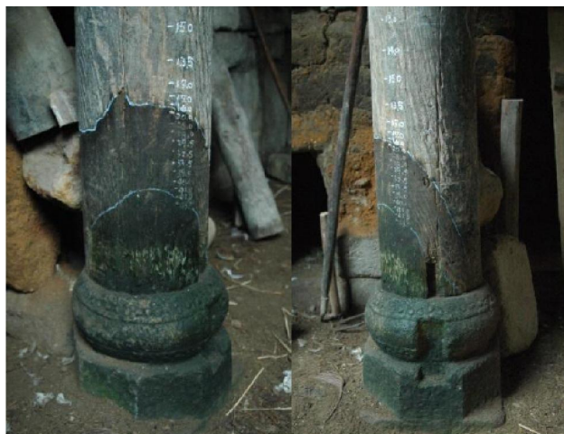
Figure 7 : Situations of the dampness pillar
