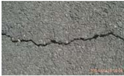
Figure 1: Original crack image figure
