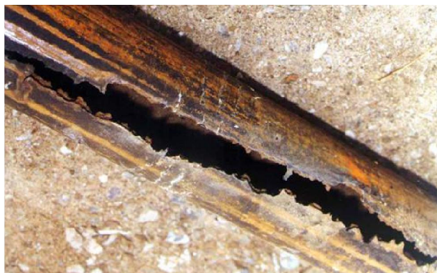
Figure 1 : The tubing corrosion in a sour gas reservoir under existence of bacteria corrosion
