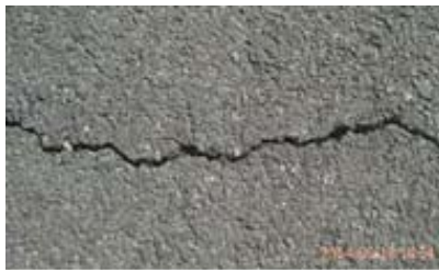
Figure 1: Original crack image figure
