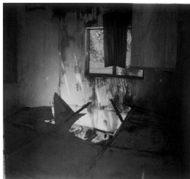
Figure 1 : Dilapidated offices in one of the state area office
